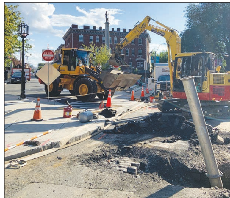
The massive Upper Broadway infrastructure and roadway project began on Monday at City Hall. Aqualine contractors will work the next two years to replace water and sewer pipes from Chelsea City Hall to the Revere line. After that, the City will reconstruct the roadway, sidewalks and drainage. The project is expected to wrap up in 2025.
