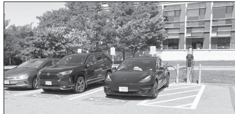
The EV charging stations at the North Shore Community College Danvers campus. EV charging stations are also available at the L
