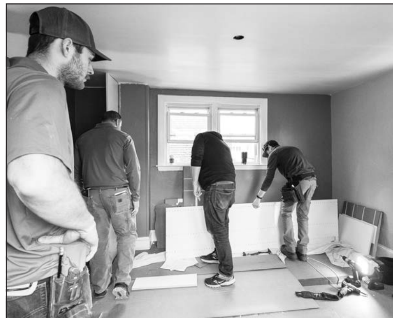
Shown above and below, team members worked hard inside and outside of Bryan's room to ensure the finished remodel was perfect.
